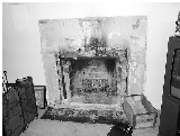
Figure 128 Ignition of wood wall-framing member from an overfired fireplace (Courtesy Tim Bradley)
